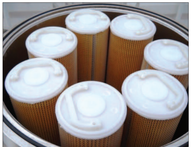
Figure 7: Inside of filter housing
