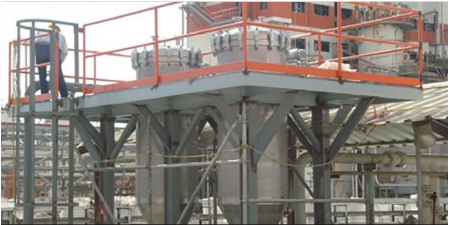
Dual Sulphurnet Self-Cleaning Candle Filter Installation
